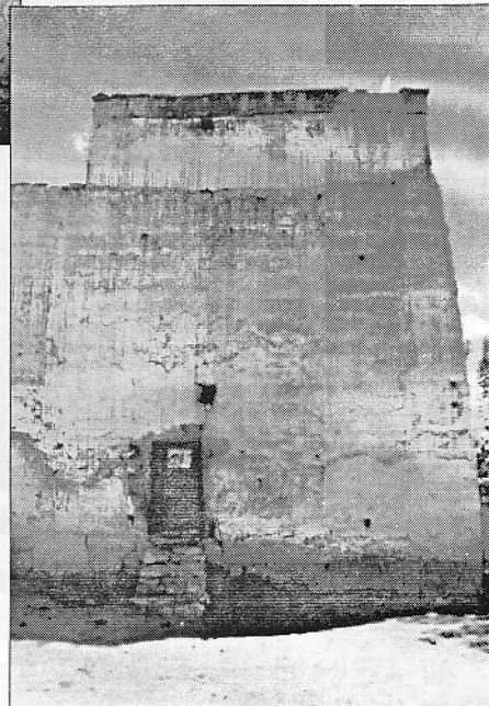
Fig 6. Illegal Puncture in town wall for private access.
