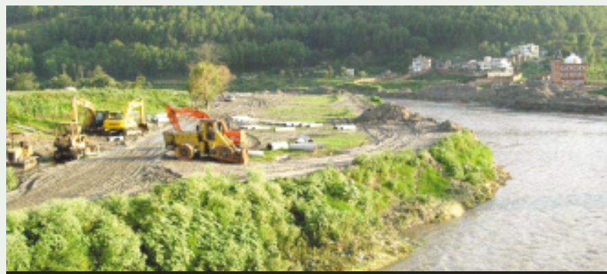
BAGMATI CORRIDOR: Bulldozers at work on the banks of the Bagmati in front of the Tribhuvan University Gate in Kirtipur
