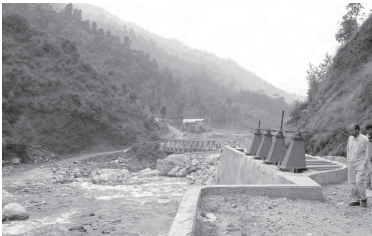
The Sun Kosi hydropower plant in Sindhupalchok built with Nepali Russian investment (above). Investor Arun Ojha inspects the intake at the plant site (left).
