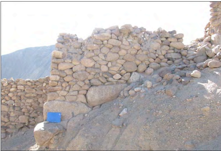
Fig. 46: Masonry of greyish cobbles at the castle of Phey. The blue folder is 24x31 cm. [credits: Devers 2009]
