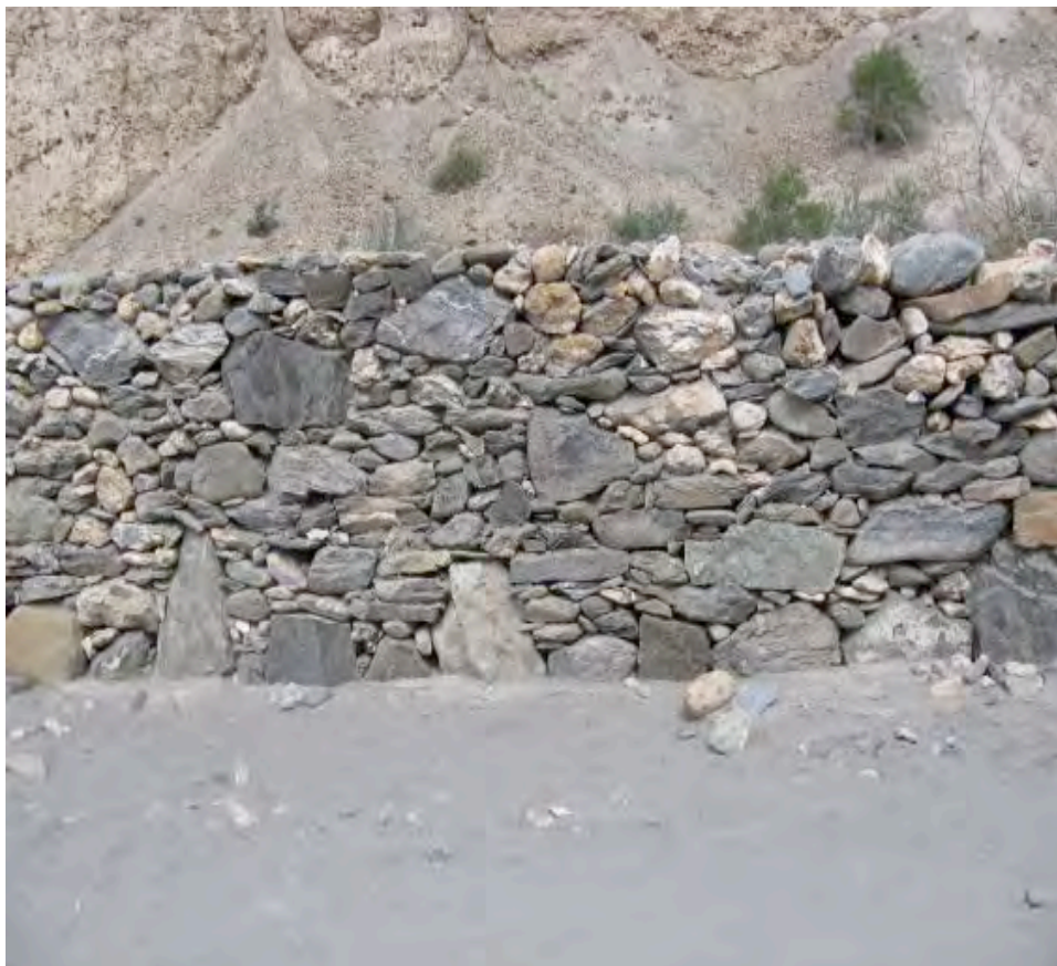
Fig. 18: Tinkle Katpa: a modern low wall using the same construction technique of stones set in the ground as a basis for the stone work. Wall in dry stone, r. 1 m high. [credits: Devers 2009]
