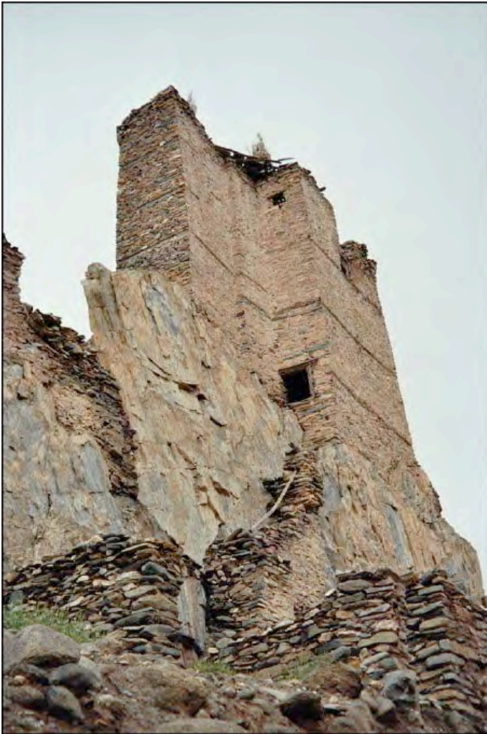
Fig. 38: Hankar: view of the tower from the south-west. Mud- mortared stones with timber lacing. [credits: Vernier 2009]
