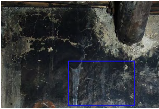
Fig. 7 — Detail of the south wall before cleaning; the blue square localize the next detail.
