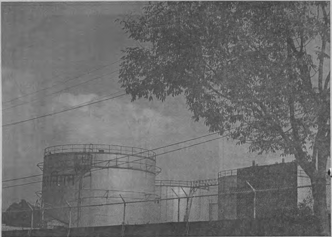
NOC's Storage Tank : Decreasing stock
